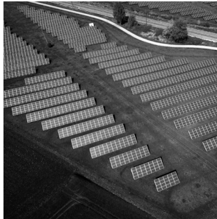
Energy Renesola pv solar farms - Poland
